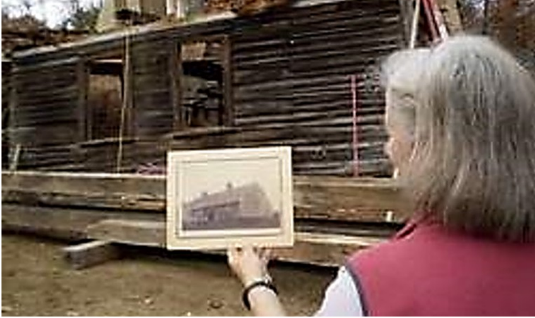
Chair Catherine Orlowicz compares a picture of the 1880 house photograph with the progress of dismantling in 2008.
