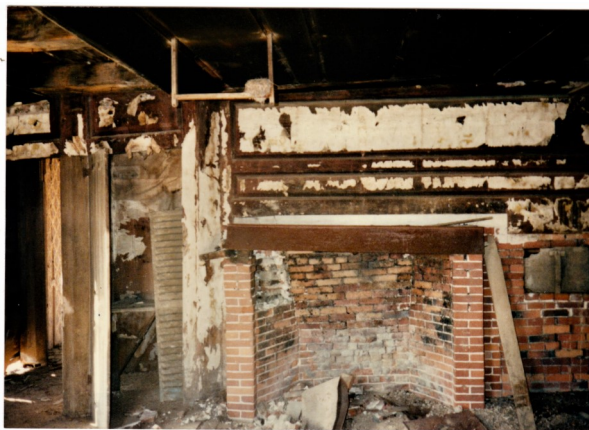
Photograph on the left is the parlor, on the right the East room fire place and bee-hive oven..
